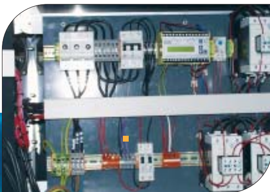
BENDER electrical safety system
