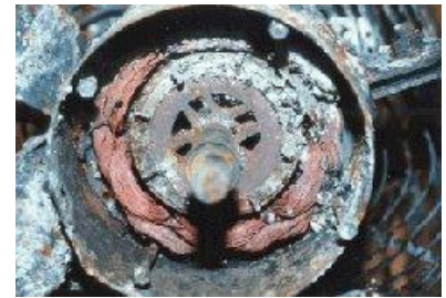
Example of Burnt Electric Motor due to Excessive Insulation Stress
